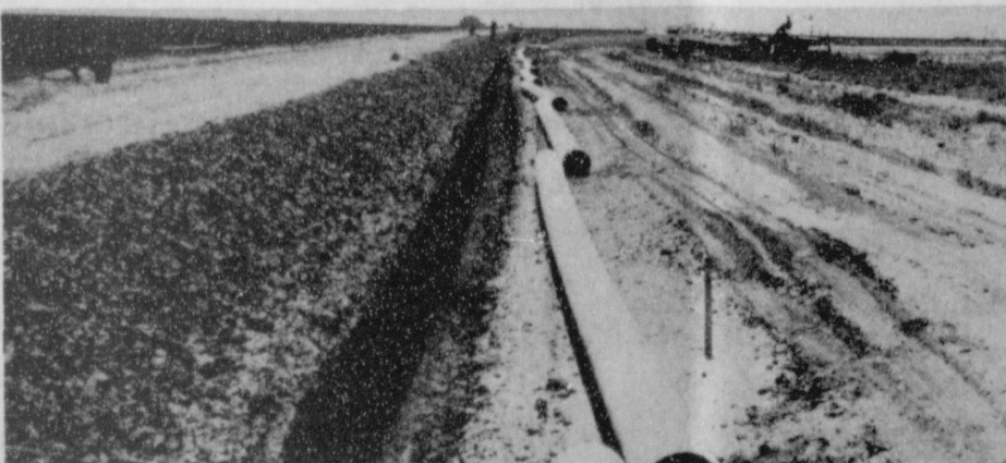
IRRIGATION PIPELINE BEING INSTALLED: Irrigation pipeline will conserve water and improve efficiency of irrigation system. The pipeline will also reduce soil erosion. Water losses on a typical ditch runs about one gallon of hour per foot of ditch or about 2.12 acre inches of water in a half mile ditchline per day. Pipeline will make it easier to cultivate and to control weeds. For further information about pipelines contact the Soil Conservation Service in Spearman.
