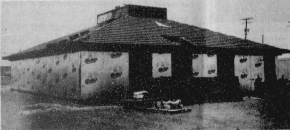
Pictured above is the new office building of Dr. Doug Steger, Optometrist. Work continued when weather permitted during the past week on the building. The building is located in the 700 block of S. Roland across from the hospital.
