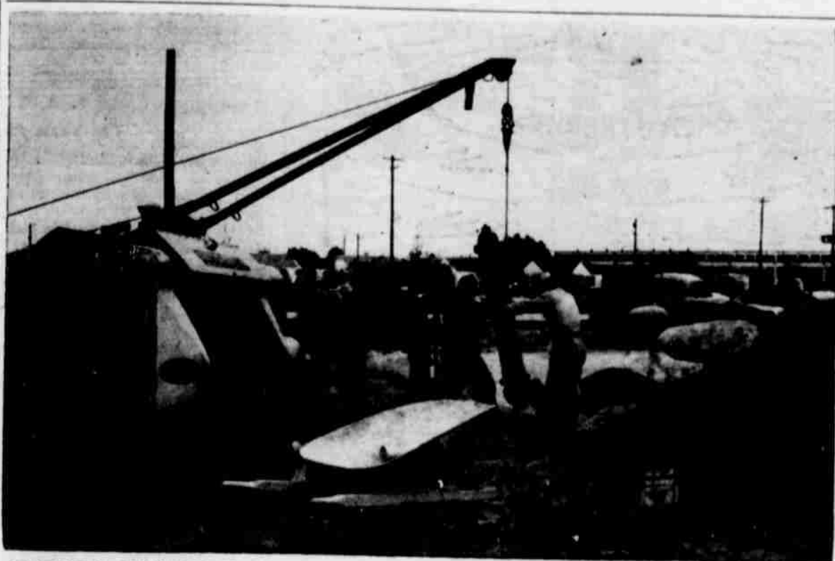
FIRE PLUG GOING IN—Shortly after the laying of new water pipe began in the southeast part of town last week, this new fire plug was erected on South Mill Street. Shown placing the plug are H. Anderson (left) truck driver, and W. E. Murray, machine operator's helper. Other workmen in the picture are digging the ditch for the new pipe.—(Staff Photo).
