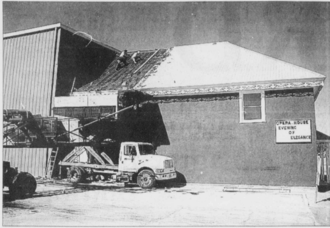
A 100 YEARS of history gets replaced as the Colorado City Opera House gets a new roof. The historic roof was damaged in June 2008 by a heavy storm cell, along with several other city facilities. Photo courtesy of City Hall.
