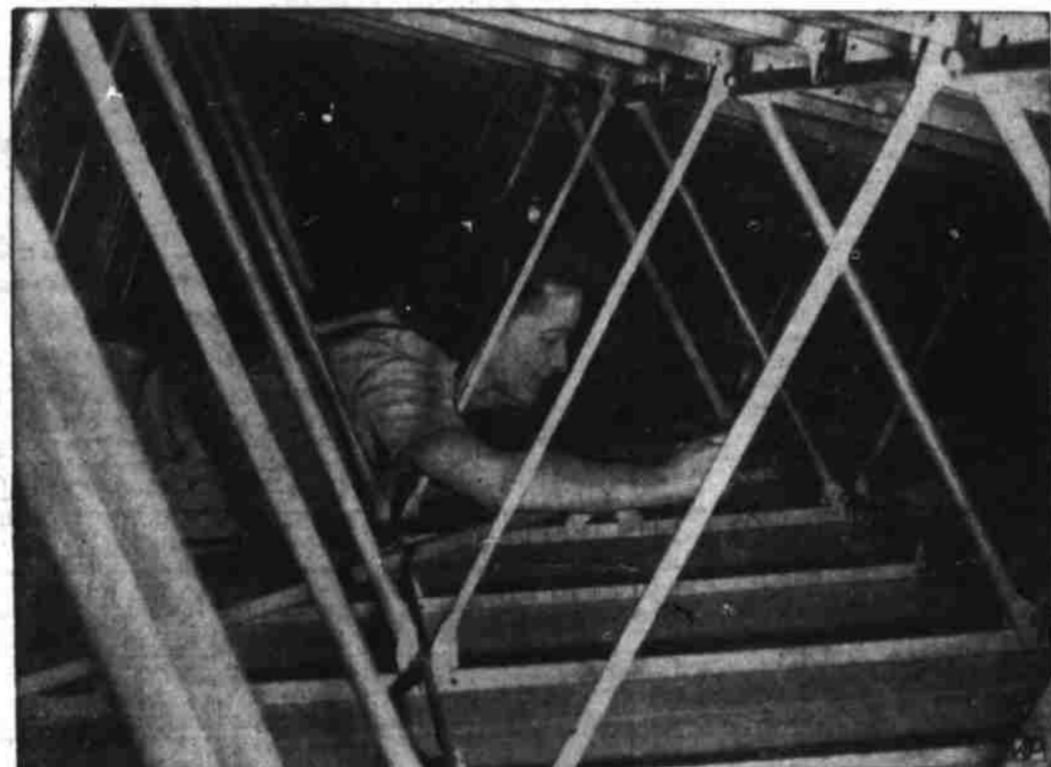
AIRPLANE SEAMSTRESS. —Inside the wing of a big clipper plane at Pan American's base at LaGuardia Field, N. Y., Marion Randall of Flushing, L. I., sews on the fabric section of the wing of the 42-ton flying boat.
