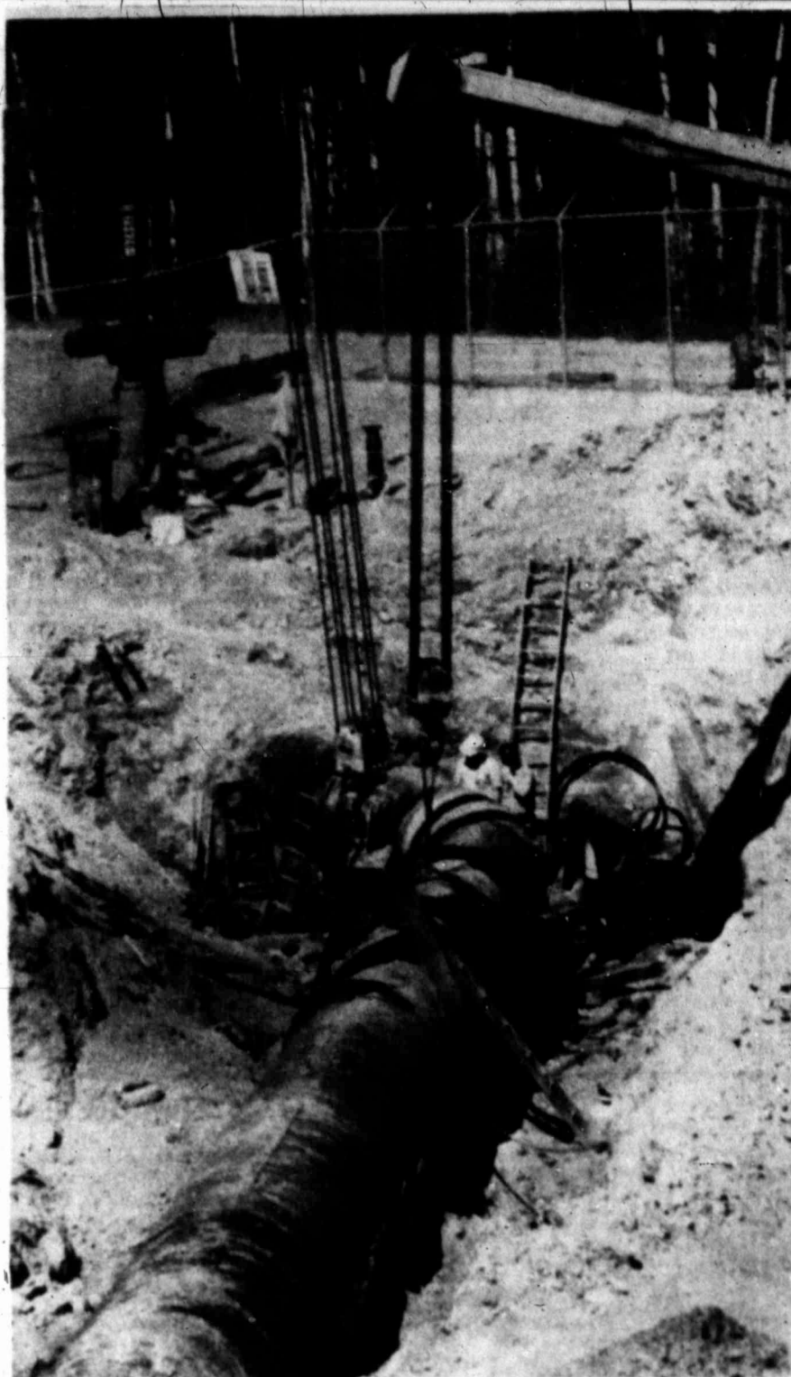
Workmen repair a cracked elbow joint which forced a shutdown of the trans-Alaska oil pipeline Monday. The crack apparently was caused by the injection of supercold liquid nitrogen instead of gaseous nitrogen into the pipe near a pump station. Gaseous nitrogen is used to purge the line of combustibles before oil goes into the line. (AP Laserphoto)
