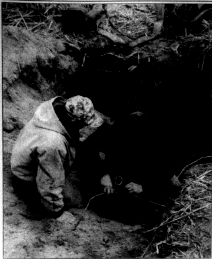
CITY WATER WORKERS Andrew Magers and Roscoe Majors work to repair a broken water line that left Subway and a local home without water for several days.
