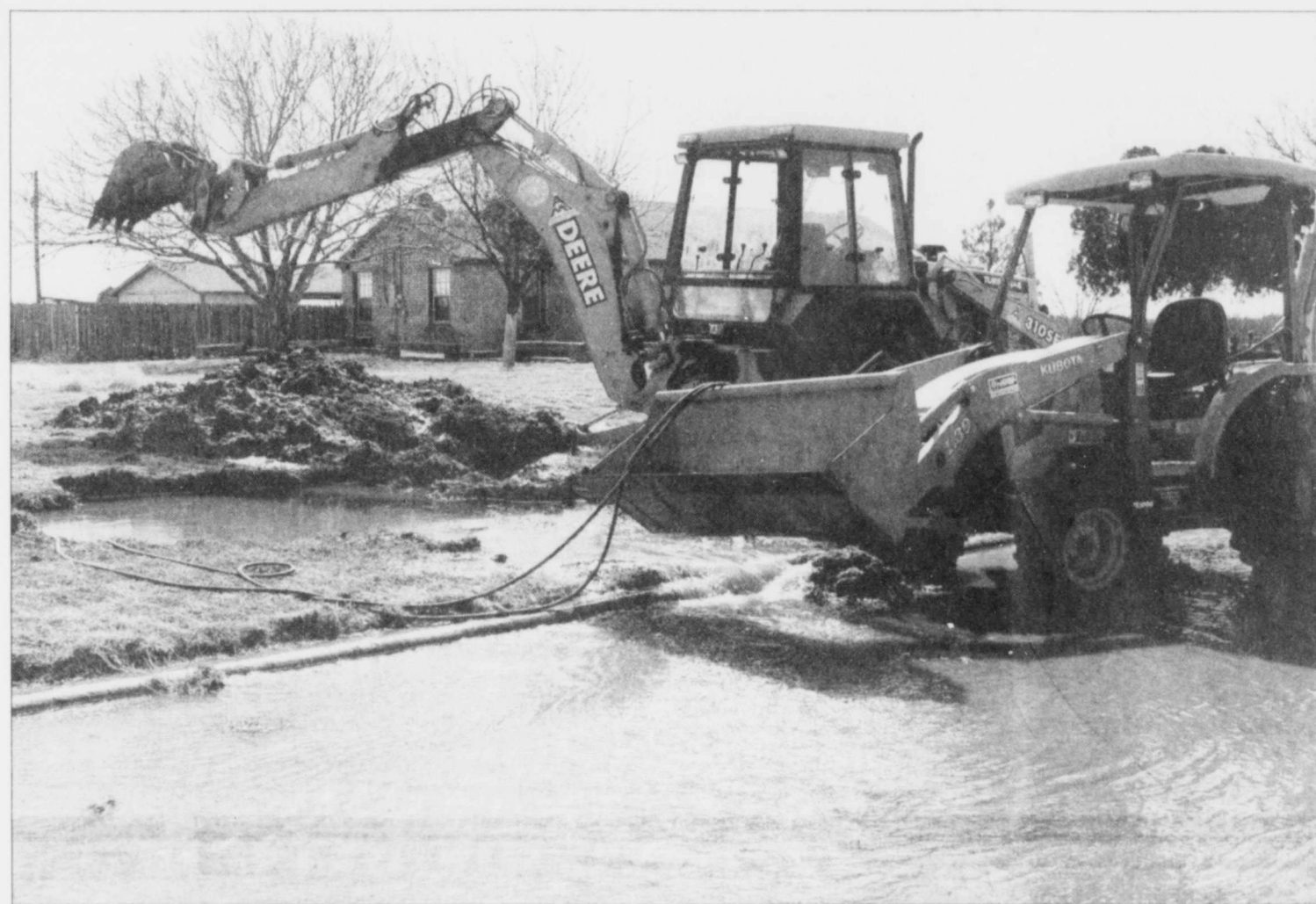
ON THE JOB -- City workers responded quickly to a water leak Tuesday afternoon on 10th Street near the Colorado City Senior Apartments. Cold temperatures, shifting soils and aging water lines combined to form sheering phase action creating breaks in the lines, according to city manager Pete Kampfer.
