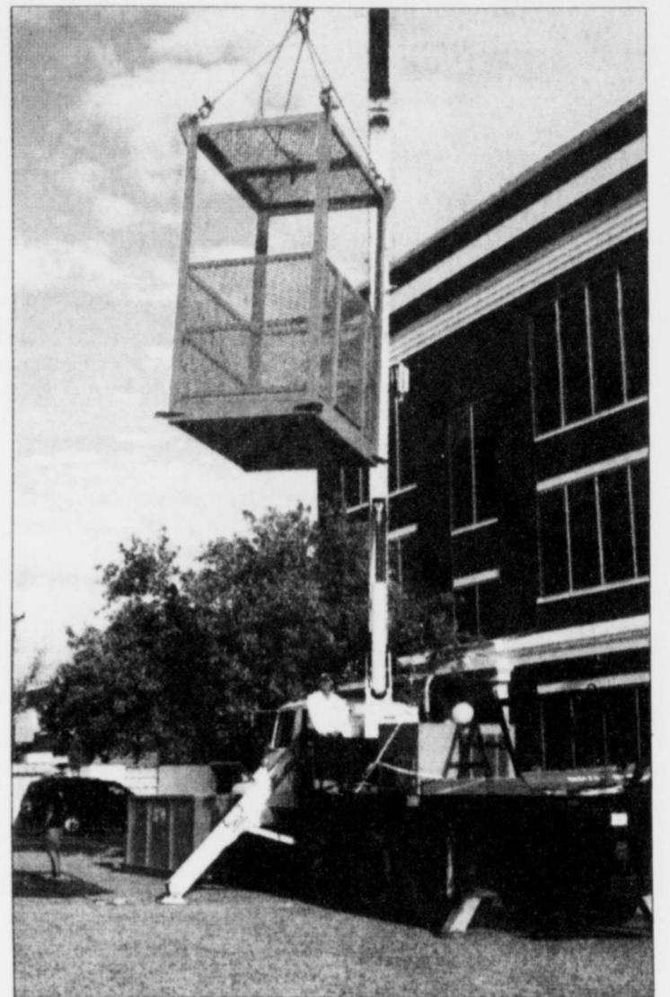
A HOIST AND BASKET, operated by Bill Ellis, was used to lower an unidentified maintenance worker who suffered severe back spasms while working on an air conditioning unit on top of the courthouse last week. Members of the DPS, Mitchell County Sheriff's Office, Colorado City Police Department, EMS, Colorado City Volunteer Fire Department responded to the scene and EMS transported him to Mitchell County Hospital where he was treated and released.
