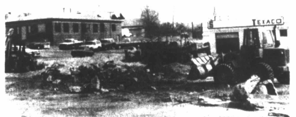
THIS IS ALL THAT REMAINS of the Mahoney Auto Parts Building located on the corner of Second and Chestnut Streets. The structure was razed to make way for additional parking space for the City National Bank and its annex.
