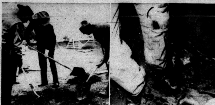
WELDING SHOVELS Tuesday afternoon are Sheriff Earl Abercrombie, Texas Ranger John M. Wood, and Mid-America Pipeline district superintendent David Luddeke. They are uncovering a well-concealed valve illegally connected to a propane pipeline. AFTER CAREFULLY UNCOVERING the line this two-valve riser was found welded into the pipe line. The feet, one standing on the main line itself, belonged to Ralph Ball, gauger foreman for the pipeline. The tap was considered a poor installation.
