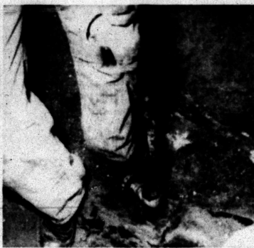
AFTER CAREFULLY UNCOVERING the line this two-valve riser was found welded into the pipe line. The feet, one standing on the main line itself, belonged to Ralph Ball, gauger foreman for the pipeline. The tap was considered a poor installation.
