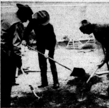
WELDING SHOVELS Tuesday afternoon are Sheriff John M. Wood, and David Luddeke, Texas Ranger John M. Wood, and Mid-America Pipeline district superintendent David Luddeke. They are uncovering a well-concealed valve illegally connected to a propane pipeline.
