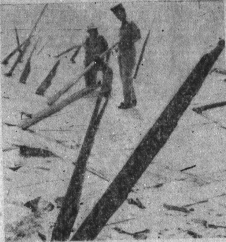
DEBRIS PUNCTURES ROOF — John Geeslin, left, maintenance man, and Capt. Jack Plemons, commander of 149th Army Aviation Company, 49th Armored Division of Texas National Guard surveys damage to hangar in Grand Prairie after tornadoes skipped through the Dallas-Ft. Worth area. (AP Wirephoto)
