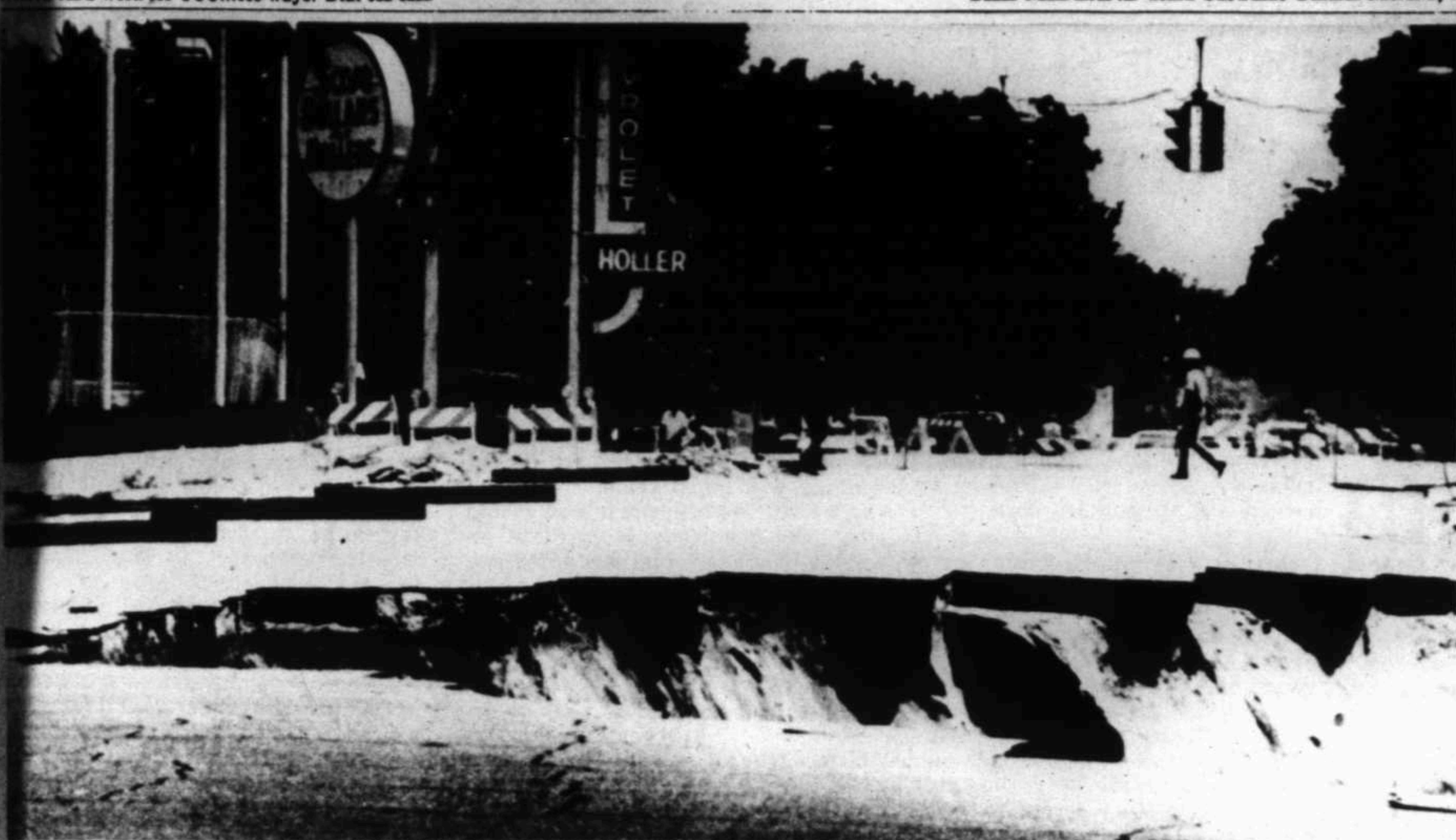
One of the roads bordering the sinkhole in Winter Park, Fla. was almost undermined as it grew about 50 feet.
