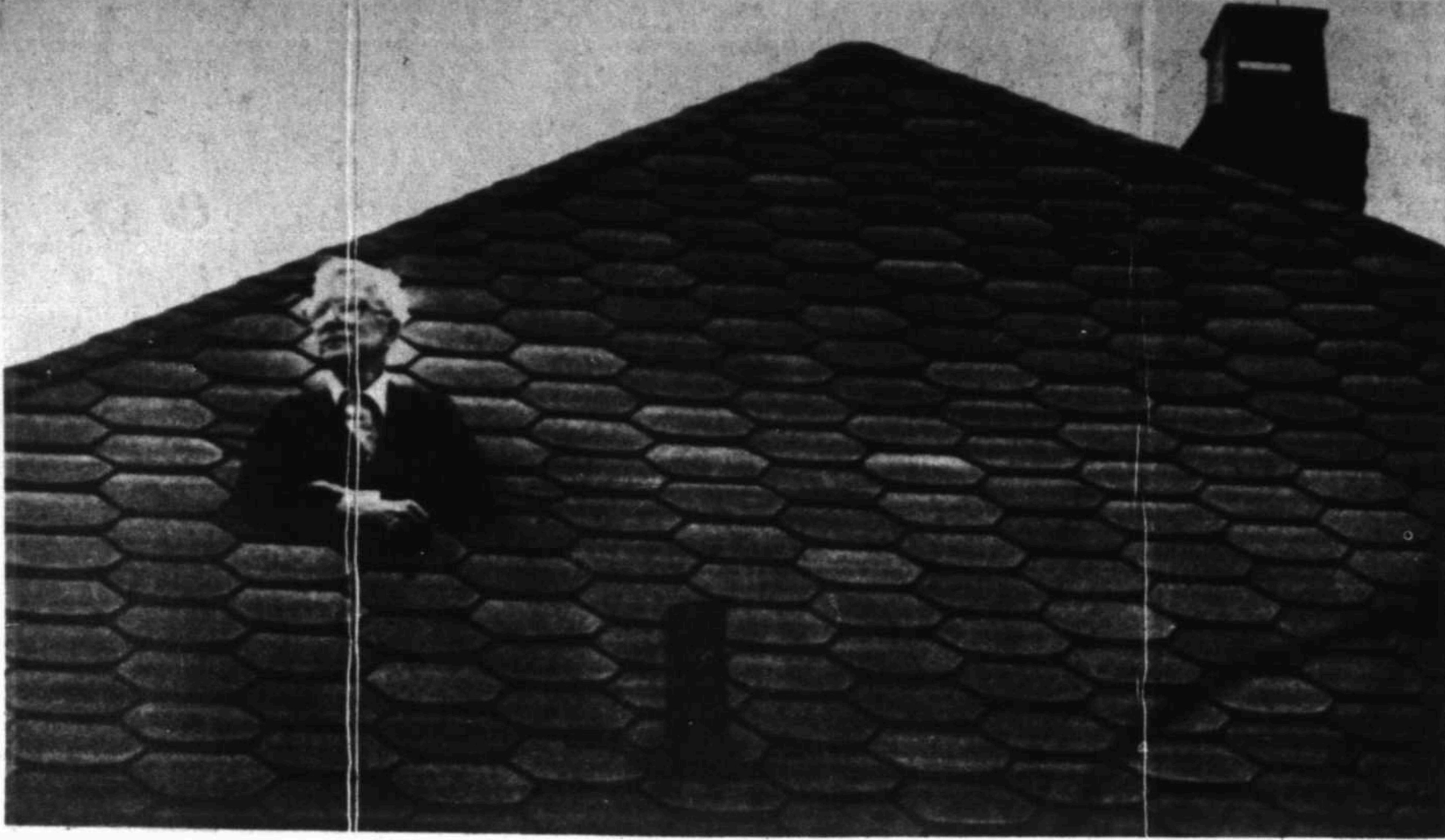
Surveying the world from the new "skylight" in his Vancouver home is Arthur Carr. The hole was provided by a falling chunk of ice, presumably from a passing airliner, which crashed through the roof Sunday.
