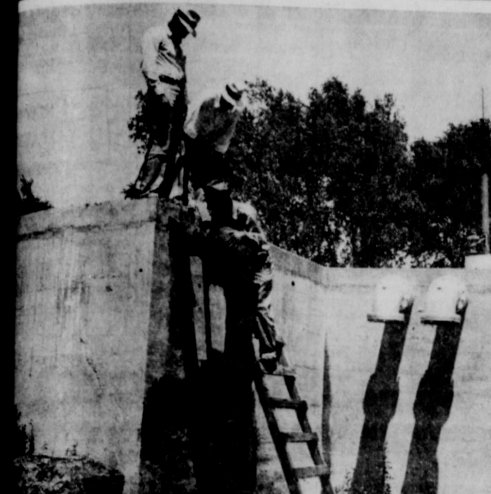
WATER LINE—This large pipe brings water from the new city well in south Perryton to the city park and will help prevent a water shortage in the hot summer months. Shown installing are J. D. Maberry, city manager J. B. Whigham, and Les Albright of the water department.
