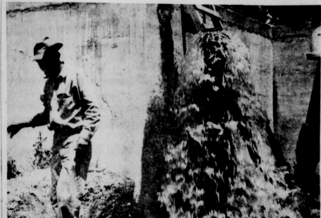
LOTS OF WATER—Comes out of this pipe from the new city well, and it was turned into the city reservoir Monday, boosting the city water capacity to around 2,750,000 gallons per day. Les Albright, left of the city water department, made the connection.
