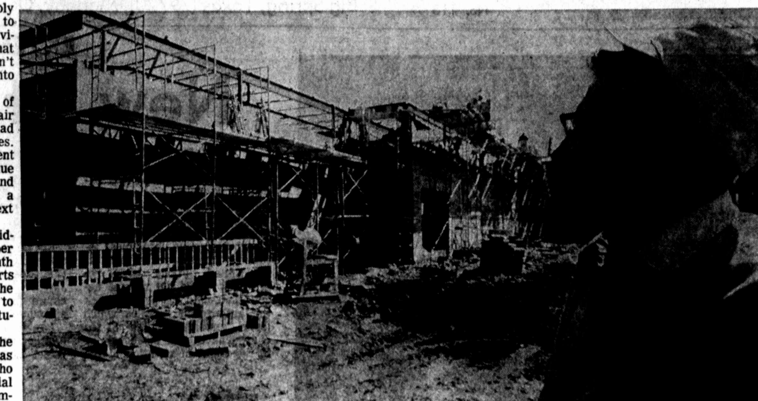
BIG JOB — Construction of a $1.6 million middle school building is a big job, but the builders hope to have the building ready for fifth to eighth grade students by the Christmas holidays.
