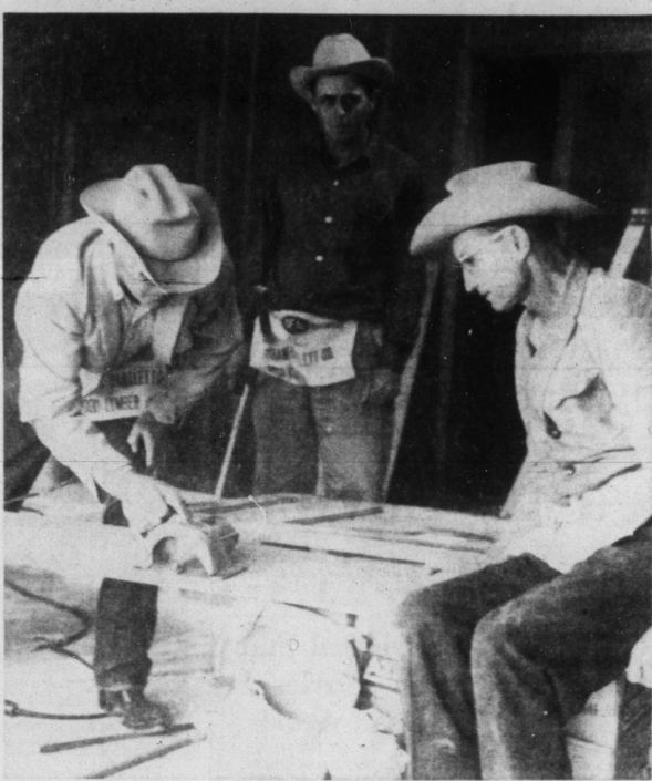
COMMISSIONERS-CARPENTER —When Scurry County commissioners discovered the budget allotment would not cover remodeling of the new Scurry County Welfare headquarters, they have to with hammers, saws and muscles to help get the old Horrell Feed Store ready for the increased allotments to be issued Feb. 8. A number of Snyder firms and individuals are contributing both materials and labor towards the renovation. From left above, are Bill Herring of Precinct No. 2; Marion Dabbs of Precinct No. 1, and J. C. Massingill of Precinct No. 4.
