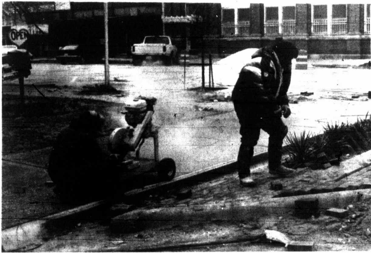
THE DOWNTOWN BEAUTIFICATION Project took center stage Friday as shrubs and trees were planted at street corners on Second Street. Enrique Anguiano and Moses Hernandez of Tommy L. Johnson Construction Co. in Shephard, Tx., cut and lay bricks.
