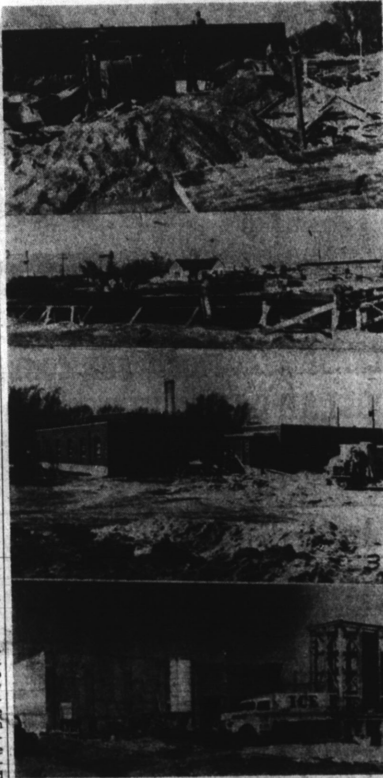
Early in February a published survey showed more than six million dollars in buildings completed, and under construction in Hereford during the past three years. Above are pictures of four public service buildings now under construction: No. 1, top, shows preliminary work on Hereford's new $335,000 hotel; 2, Forms are being run on the new $475,000 Shirley School to accommodate the influx of pre-Junior High students; 3, The new $285,000 Deaf Smith County Hospital annex is nearing completion, and picture No. 4 shows the new $50,000 ice plant, also nearing completion.
