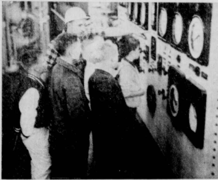
THE OPERATIONS OF the turbine control panel at Tuco are explained by Maurice Tow, Tuco employee, as a group of local seventh graders look on. The photo was made during National Electrical Week when three groups of local seventh graders toured the plant facilities. Groups of students from Petersburg and New Deal Schools visited the plant during the following two weeks.
