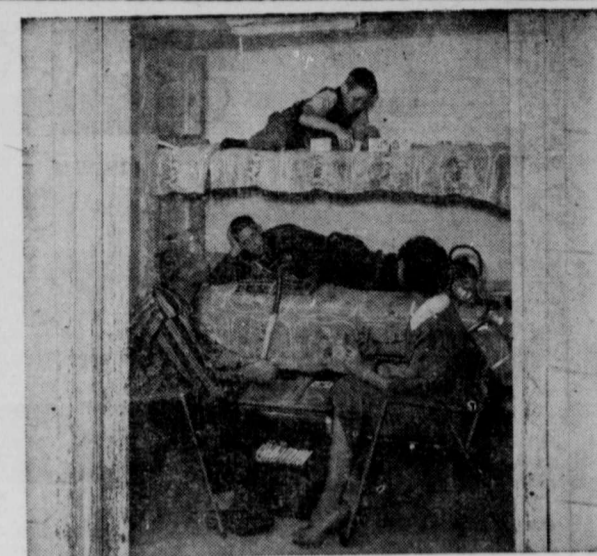
A CLOSE CALL with a tornado in 1953 led the Donald L. Anderson family of Toledo, Iowa, to build their own small shelter adjoining their basement. They estimate that, by doing their own work, they will have only about $50 in the shelter when finished. Here Anderson, his wife Jean, and sons Rick, 13, (lower bunk) and Don G., 12, "try the shelter out for size." In addition to serving as a tornado shelter, it would be valuable as protection against radioactive fallout if the nation were attacked. (OCDM Photo)
