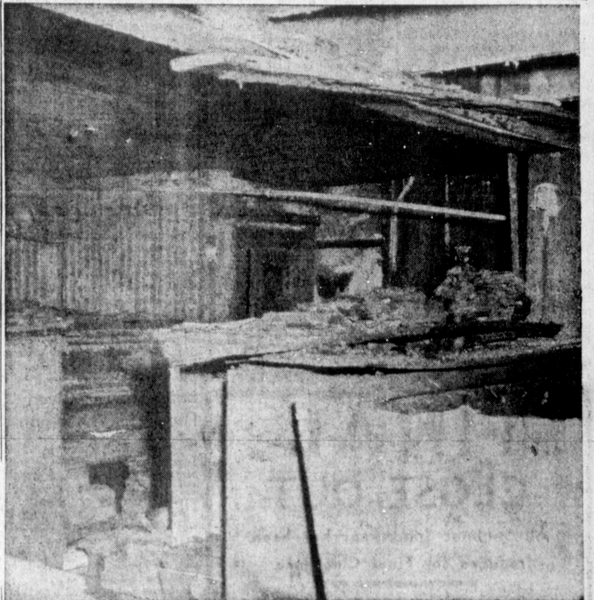
HEAVY DAMAGE — Shown is part of the interior of Ard Music Store, located at 115 N. Cuyler, which received heavy damage from a fire of undetermined origin last night. The fire was discovered at approximately 11:40 p.m. Thursday. (News photo)
