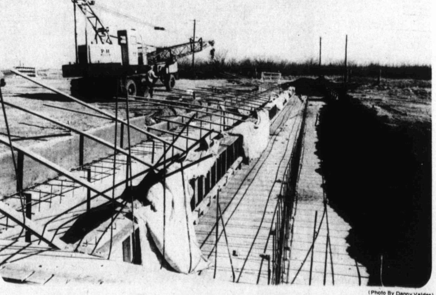
EXTENDING CULVERT — Workers prepare to extend newly enlarged culverts across the east lane of U.S. 87 north of Big Spring. In addition to rebuilding part of the east lane, the west lane will be resurfaced. Price Construction Inc., Big Spring, and Zack Burkett, Graham, have contracted to perform the work on 1.6 miles of highway for $540,985. A.J. Dean, Texas Highway Department engineering technician, said. The project is expected to be complete in the fall.
