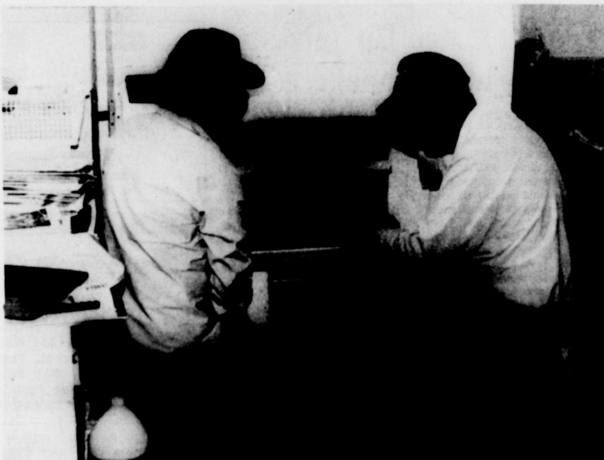
COLORADO ISD maintenance employees Luis Molina (left) and Clarence Freeman are checking air conditioning units at Colorado Middle School in preparation for the first day of school which is August 18. Teachers report for work on August 12th.
