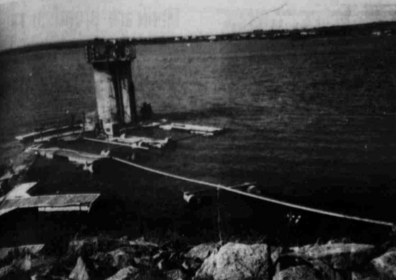
DREDGE PUMP OPERATION — A dredge pump, "ported" from Houston, is shown in the above picture as it works to clean out the filtration plant's intake pipe at White River Lake and end the water emergency. The dredge pump is the
