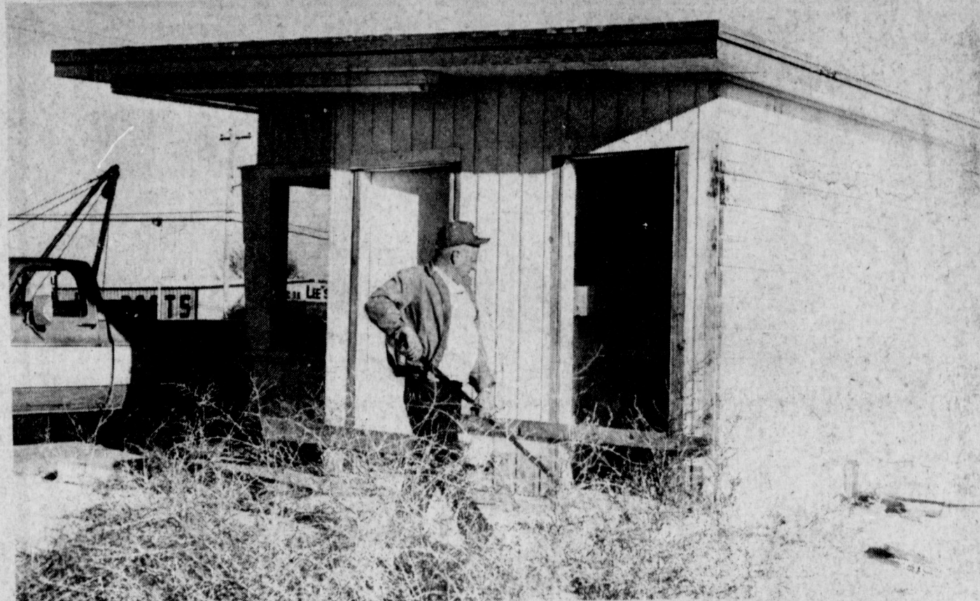
GETTING READY TO MOVE --Several men were at a location on west American Blvd. Monday afternoon to move a small building to the Muleshoe Youth Activities Committee miniature golf course. The building was donated to YAC by Steve Stephens, owner of Town and Country Food Stores, who will be constructing a new food store in Muleshoe in the near future. The former service station will be remodeled to be used as a ticket office, concession stand, storage area at the golf course.
