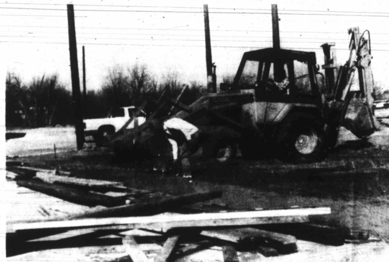
CONSTRUCTION ON THE NEW TACO JOHN'S AND SUBWAY restaurants is expected to be completed by mid-March, according to Junior Heidelberg, owner of West Texas Building Systems out of Stanton. Heidelberg, operating the tractor, and Gus Pardon were out Friday afternoon trying to finish up some dirt work at the site.
