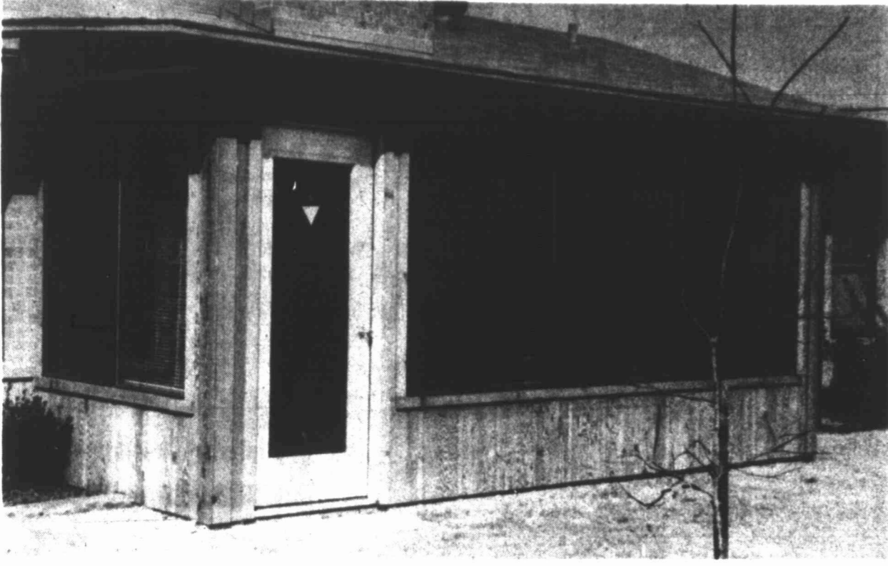
This sunny den with woodburning fireplace is a custom room addition designed and constructed by Bob's Custom Woodwork. For room additions or garage conversions, the firm carefully matches
