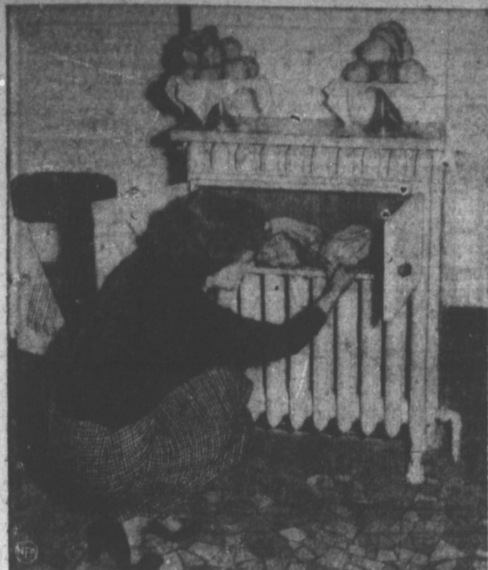
DINNER COLD? CALL THE JANITOR —Built into homes and restaurants in Florence, Italy are these double-purpose radiators, which contain a food-warming compartment. Cynthia Chaparran of Cleveland, Ohio, takes a peek to see how roast chicken's coming.
