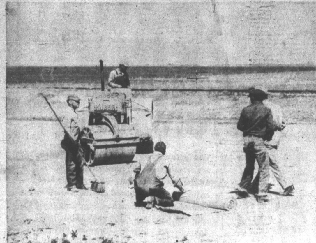
DOWN SHE GOES and a new road bed is formed. Workmen are shown above rolling the new asphalt topping to a portion of State Highway 152, inundated by the 1950 floods, which has been raised two feet above the high water level of the flood. The work is being done in four spots on State 152 and at one point along U.S. Highway 60, east of Pampa, at a cost of $108,000. (News Photo)
