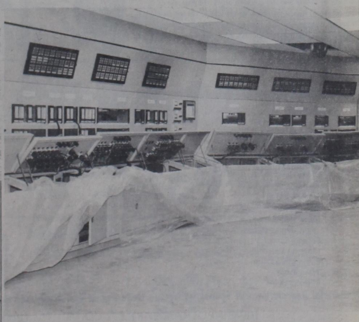
THE CENTRAL CONTROL ROOM in the new refinery at the Dimmitt Amstar Plant will electronically monitor every phase of the refining process. A six-week test of electrical
