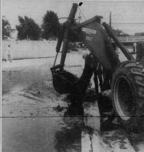
DEBRIS IN DEEP CREEK—City employees were kept busy this morning keeping the "whistler" type culverts under the low-water bridge on Twenty-eighth Street open. Two of the five six-foot tunnels were blocked at the time this picture was taken, and water on the upstream side was nearly three feet above the downstream side. Water had not crossed the bridge at noon, but City Engineer Bill Kinney said any more showers on the Deep Creek watershed would certainly send water over the bridge.
