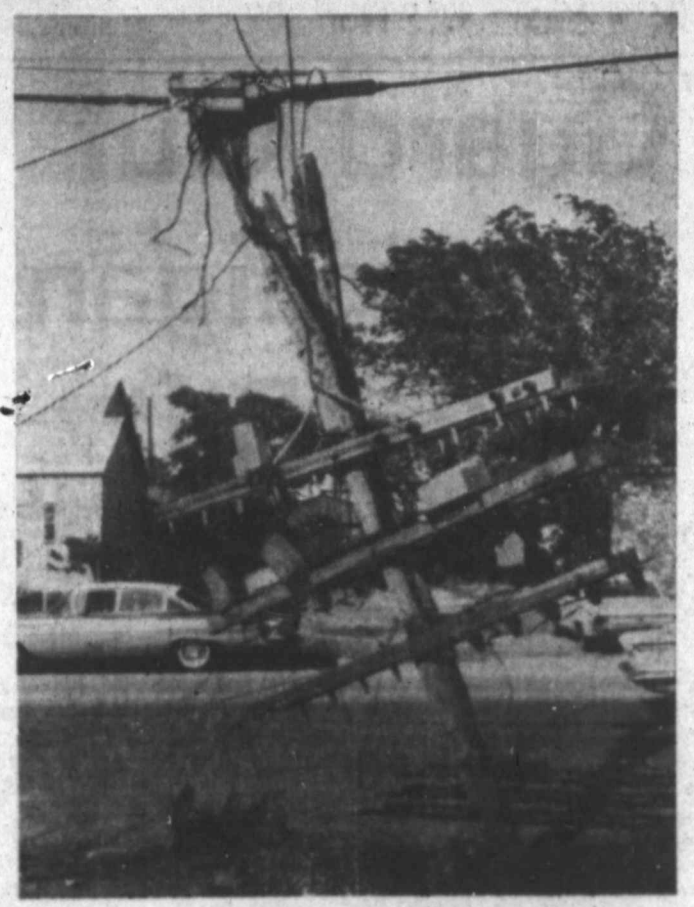
POLE SMASHED South of east viaduct
