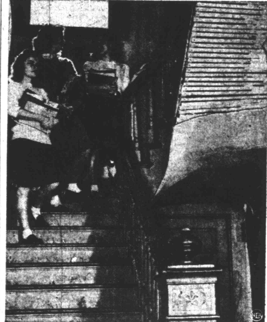
An old residence is a make-shift school building for these Alabama children. Stairways are narrow and inadequate; crumbling plaster (upper right) is an ever-present danger.
