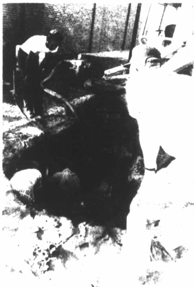
A LEAK IN THE WATER MAIN on the corner of Second and Elm Streets caused water to spout five feet into the air about 5:30 a.m. Saturday. City Water Superintendent Buzz Rich (left) and his crew worked into the week to correct the problem. The water flow from the leak was stopped about noon on Saturday but it was necessary to order a new fitting for the pipe so the open pit remained open until Tuesday.
