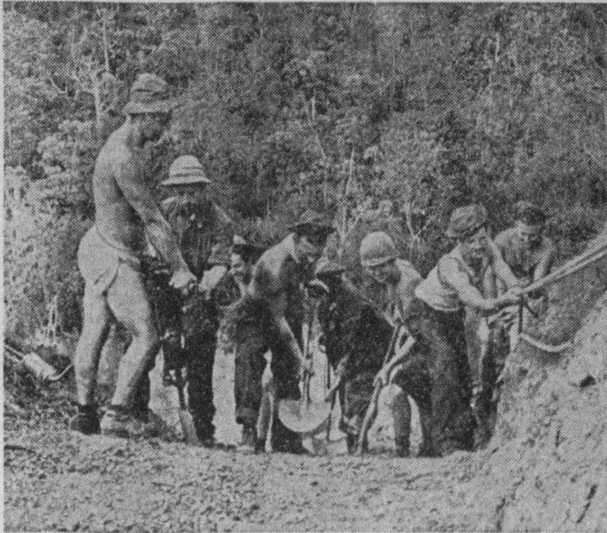
Building "Pee" roads in New Guinea is all part of the day's work for American army engineers. This particular road under construction near Port Moresby, main Allied base in New Guinea, is so steep that the men must hold on to ropes to keep from falling backward. The grade drops about 65 degrees behind them.
