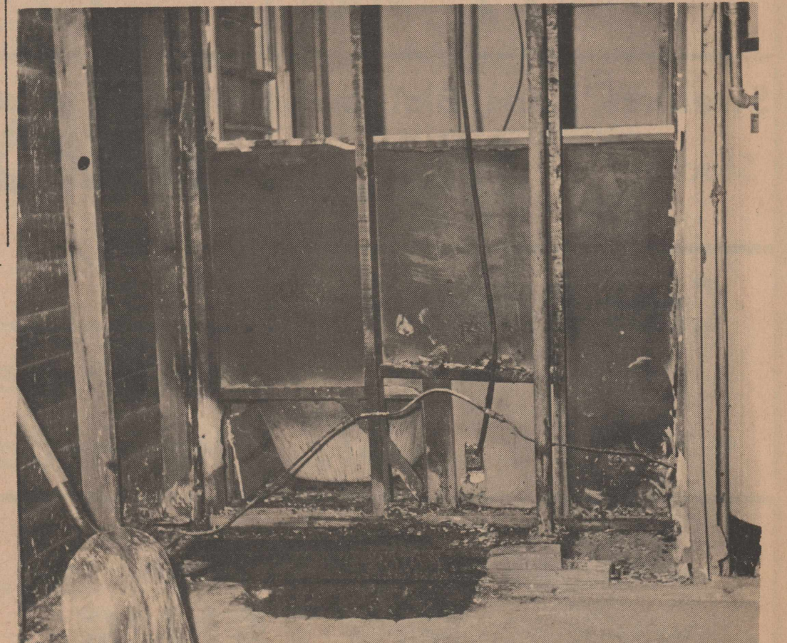
WHERE FIRE STARTED—This hole in the flooring marks the spot where clothes, set on fire by a leaking butane line, fell, starting a fire which heavily damaged the George Brown Sr. residence north of Circle. In the background is the line believed to have been the culprit in the fire.
