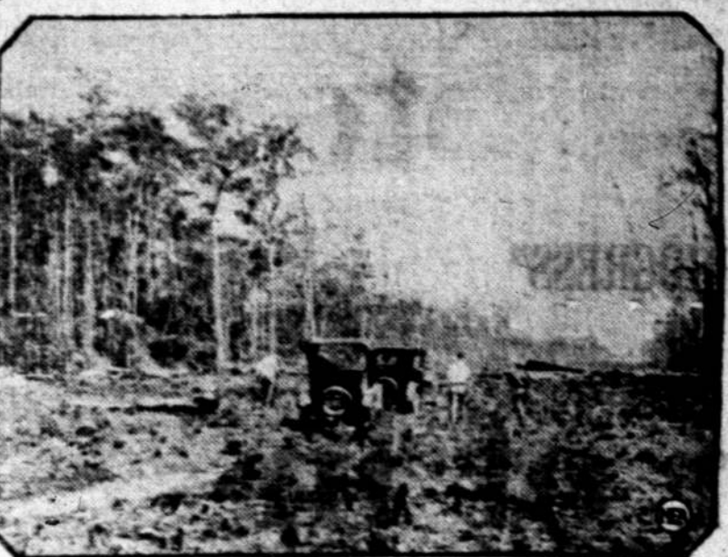
This bleak, trackless waste in the Florida Everglades will be converted into fine road crossing the state by next spring.
