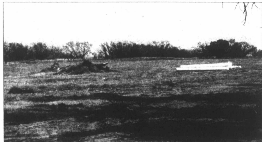
EXTENDING SERVICE - The City of Colorado City is in the process of having a water line installed that will eventually connect to a new water tower north of town. This pipe is laying near the site of the planned Best Western Inn & Suites, as the line has been bored under N. Hwy. 208.
