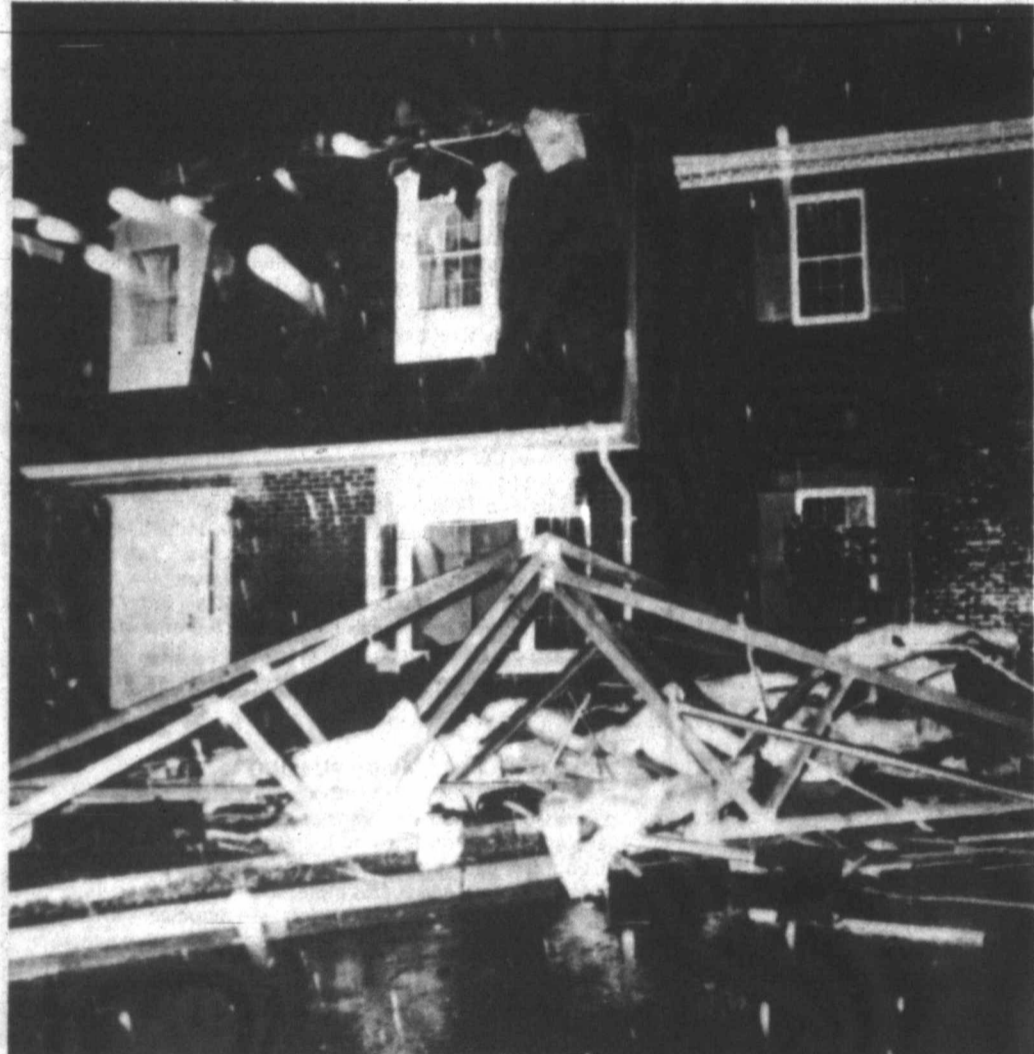
HIGH WINDS associated with Hurricane David tore this roof from a house in Fairfax County, Va., Wednesday night. The storm ripped across the northern Virginia area causing minor damage and some flooding. (AP Laser photo)
