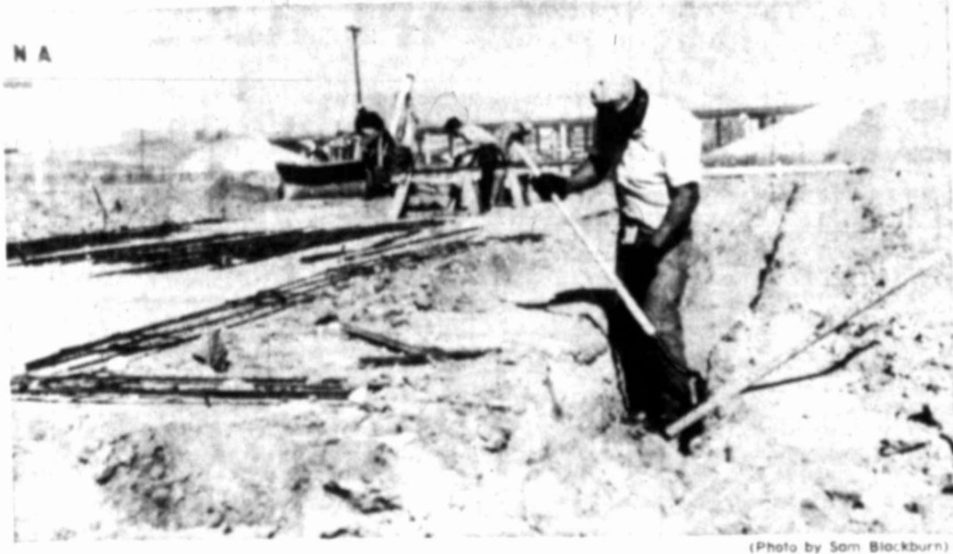
HOLIDAY INN BEGINS WORK ON APARTMENT COMPLEX Workmen prepare site for construction of eight rental units
