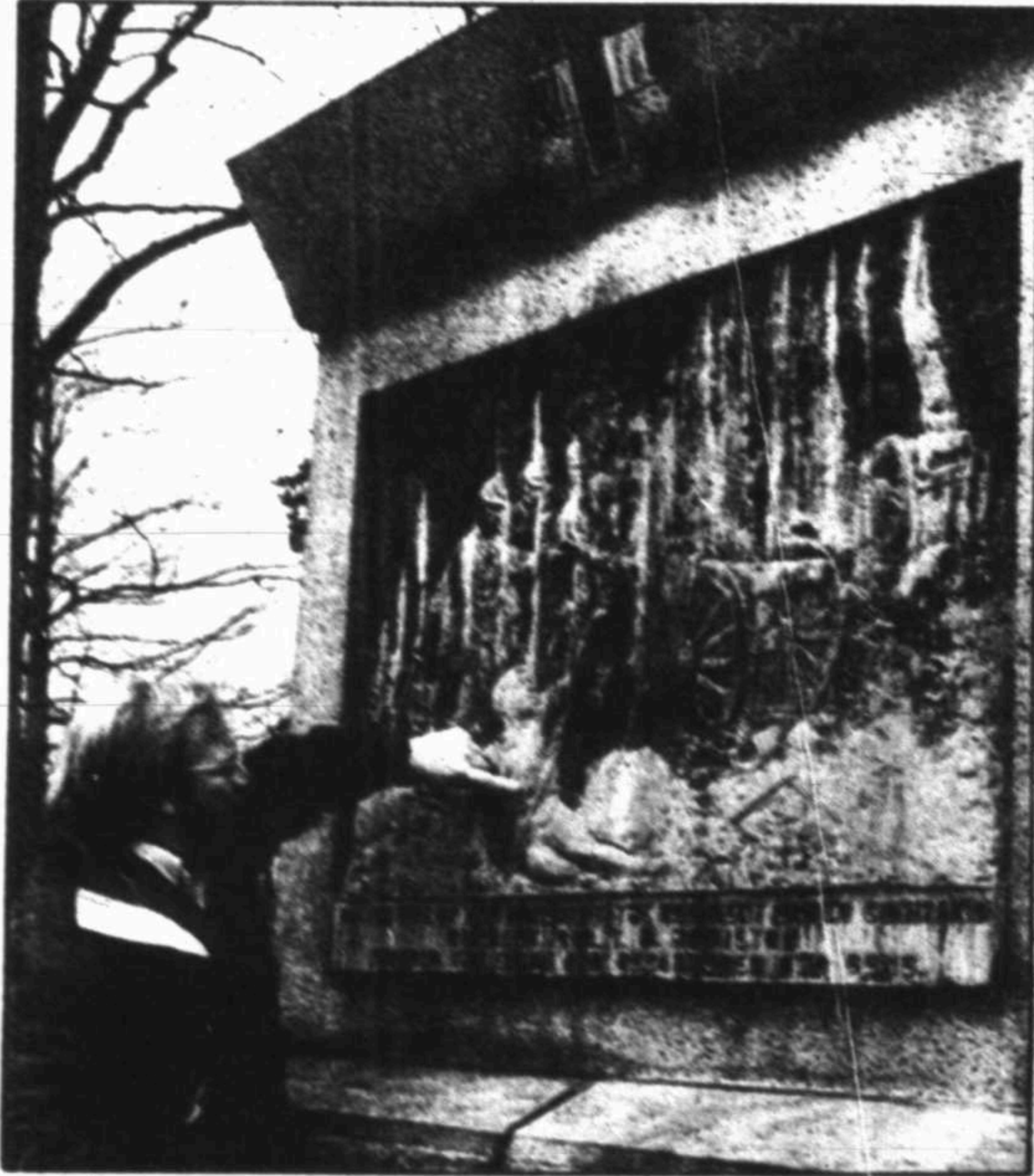
David Ballard, maintenance director at the Gettysburg National Military Park, displays the damage caused by acid rain to the 62nd New York Infantry Monument on the edge of the Gettysburg, Pa.
