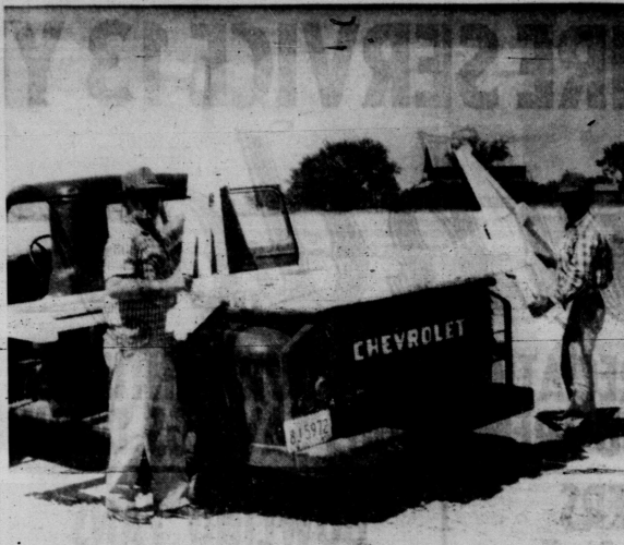
FOR SAFETY'S SAKE—B. C. McKinzie and Shorty Bevers, employes of C. H. C. Company, are shown unloading supports for the barricades on the new section of the Highway 180 by-pass. C. H. C. is the contractor on the job, and will start laying the base material for the paving in a few days. In addition to "Road Closed" signs, other good advice signs such as "Drive Carefully—Construction" and "Observe Warning Signs" are being erected. A guard rail will also be erected at the northwest end of the project to keep traffic safely on the detour portion.
