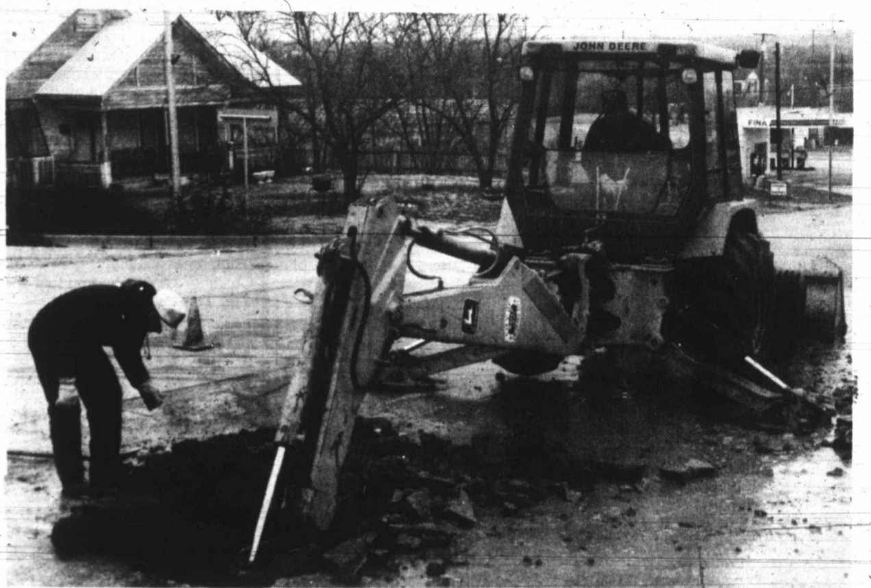
CITY WATER MAINTAINANCE EMPLOYEES WERE OUT IN THE COLD this week as they repaired several waterlines that broke because of the freezing weather. These waterlines are among those scheduled for replacement in the city's water and sewer project.
