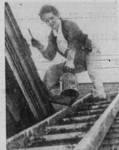
GREAT-GRANDMOTHER AT WORK—Mrs. Adoh Whitcomb, who'll be 70 this month, goes up on the roof of her three-story nursing home, in Rochester, N. Y., to fix chimney and slate shingles as she has done four times this year. She also put two coats of paint on her double garage, mixed 900 pounds of cement and floor'd fruit cellar, built a back porch and mows the lawn regularly. She has "five or six great-grandchildren." (AP Wirephoto)
