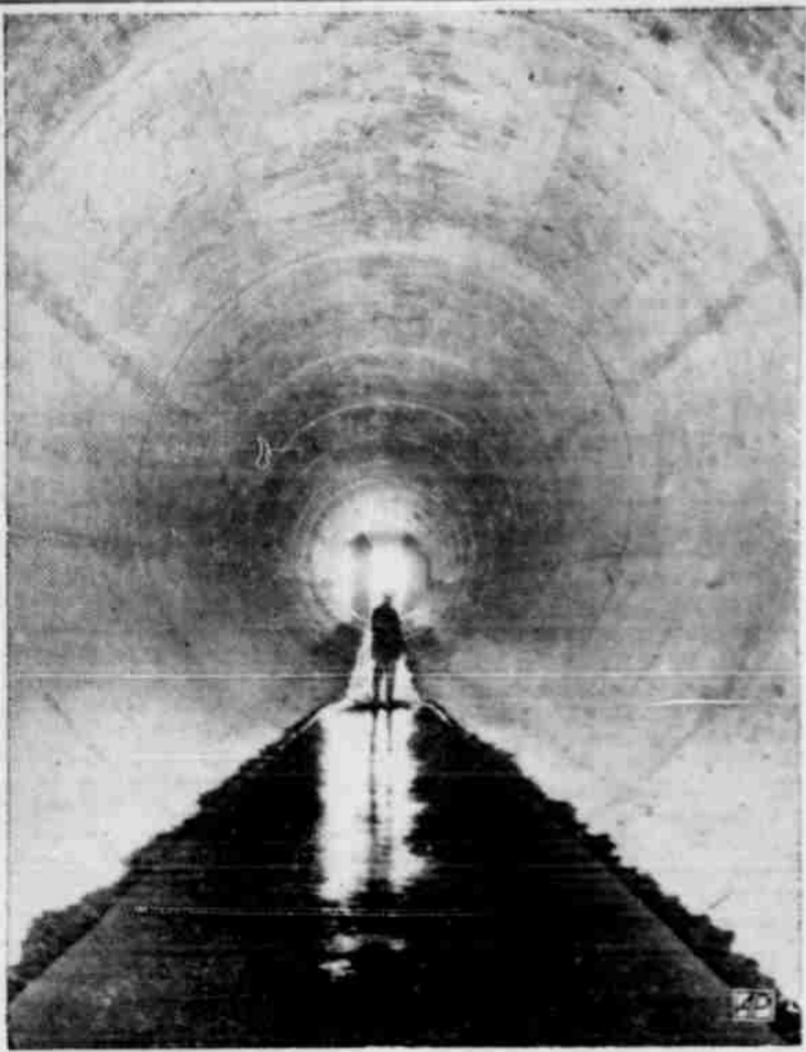
WATER CONDUIT — The six-foot man is dwarfed in one of the two 18-foot conduits under the North Concho River dam tributary near San Angelo. In time of flood, these conduits would be full of water. The dam will be nearly completed March 15, 10% months ahead of schedule. (AP Photo).
