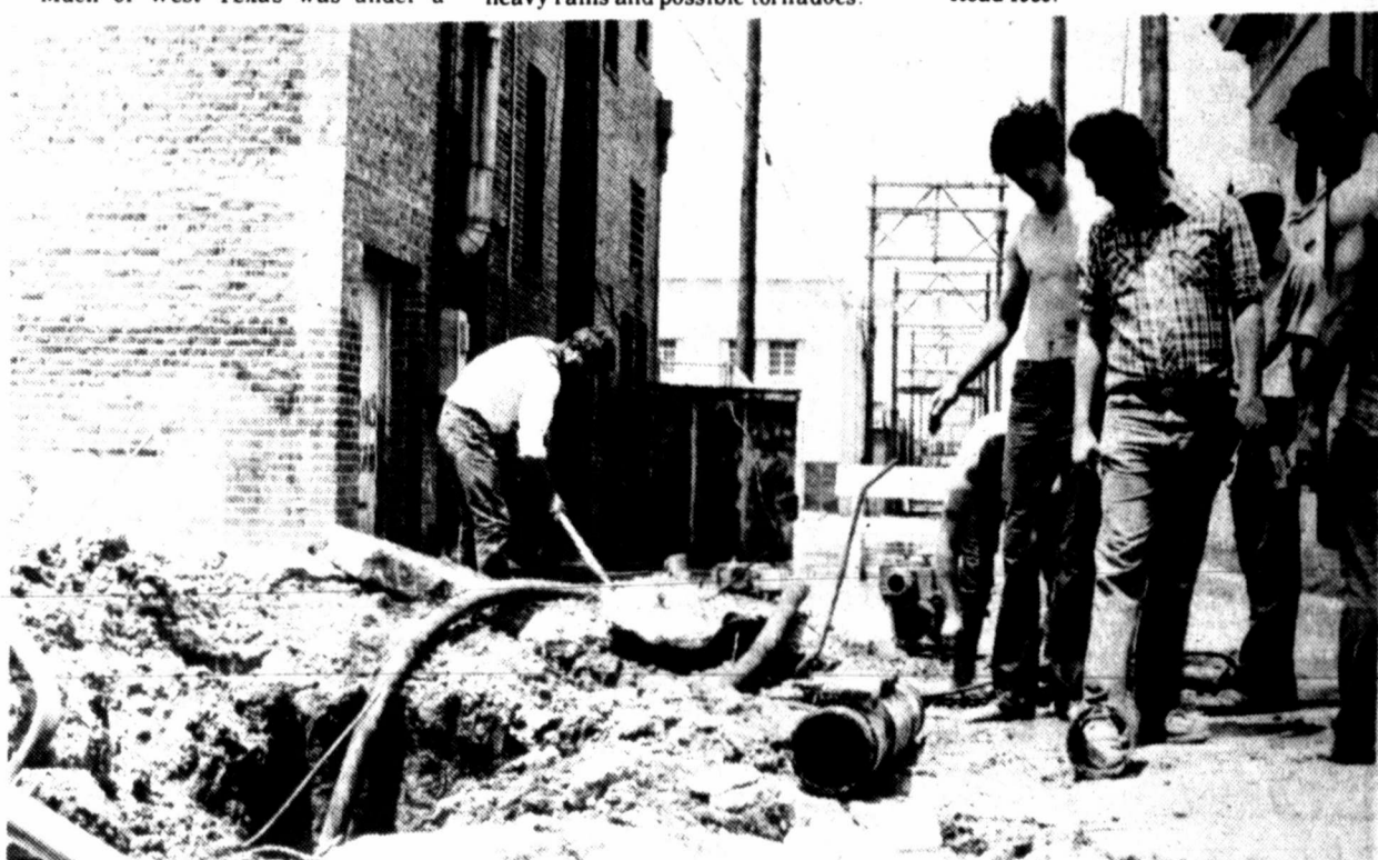
WATERLINE BREAK. City crews worked most of the day Tuesday to make repairs at a break in a downtown six-inch water pipe. The break occurred in the alley between
