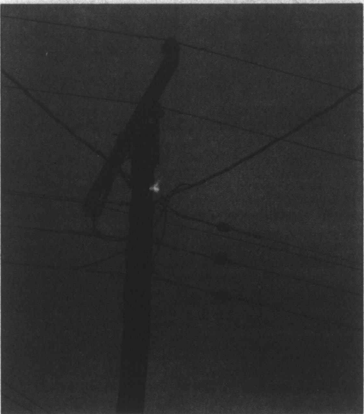
A VICTIM OF THE STORM? This telephone pole on Cypress St. caught fire Monday morning, and members of the Colorado City Volunteer Fire Department were called to put it out. A retired employee of TXU said that lightning probably struck the pole causing the blaze.
