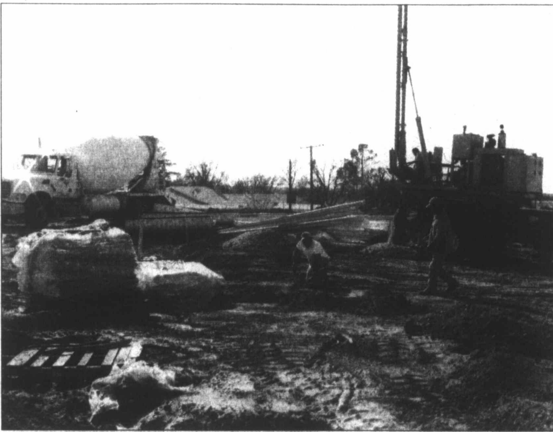
HOTEL GOING IN - Concrete piers were being poured at the site of the planned Super 8 Hotel on Monday. Developers say that the foundation work is expected to begin in a week or two.
