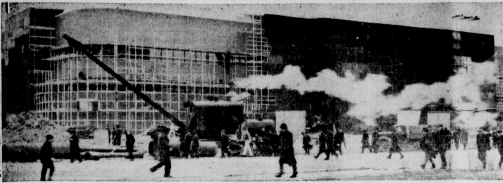
Workmen have begun tearing down the huge fiberboard canopy which sheltered the $21,000,000 Ford airplane engine plant at Dearborn, Mich., during winter construction. This view shows the front section of the plant. The entire building will be completed early in
