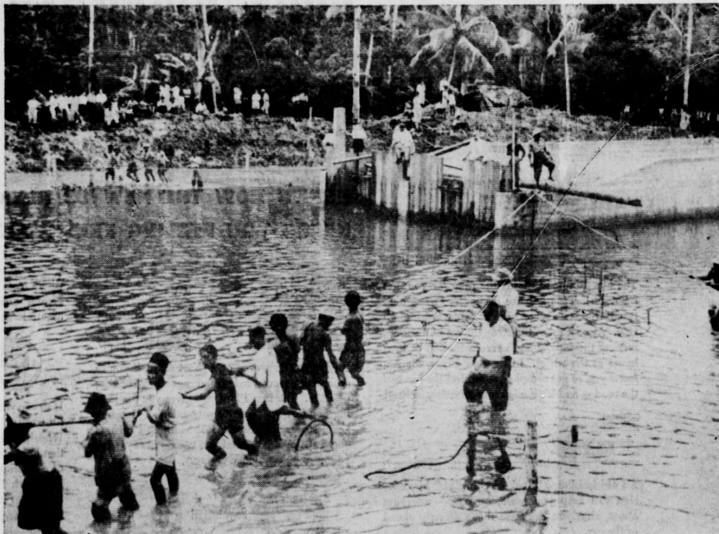
FOR DRAINAGE —A 540-ton drainage-control gate is being towed into position by workers on the Sri Menanti project to protect some 42,400 acres of agricultural land at Kuala Lumpur, Malaya. Probably the largest of its kind in Southeast Asia, the gate is made of reinforced concrete, is 123 feet long and measures 27 feet in width.
