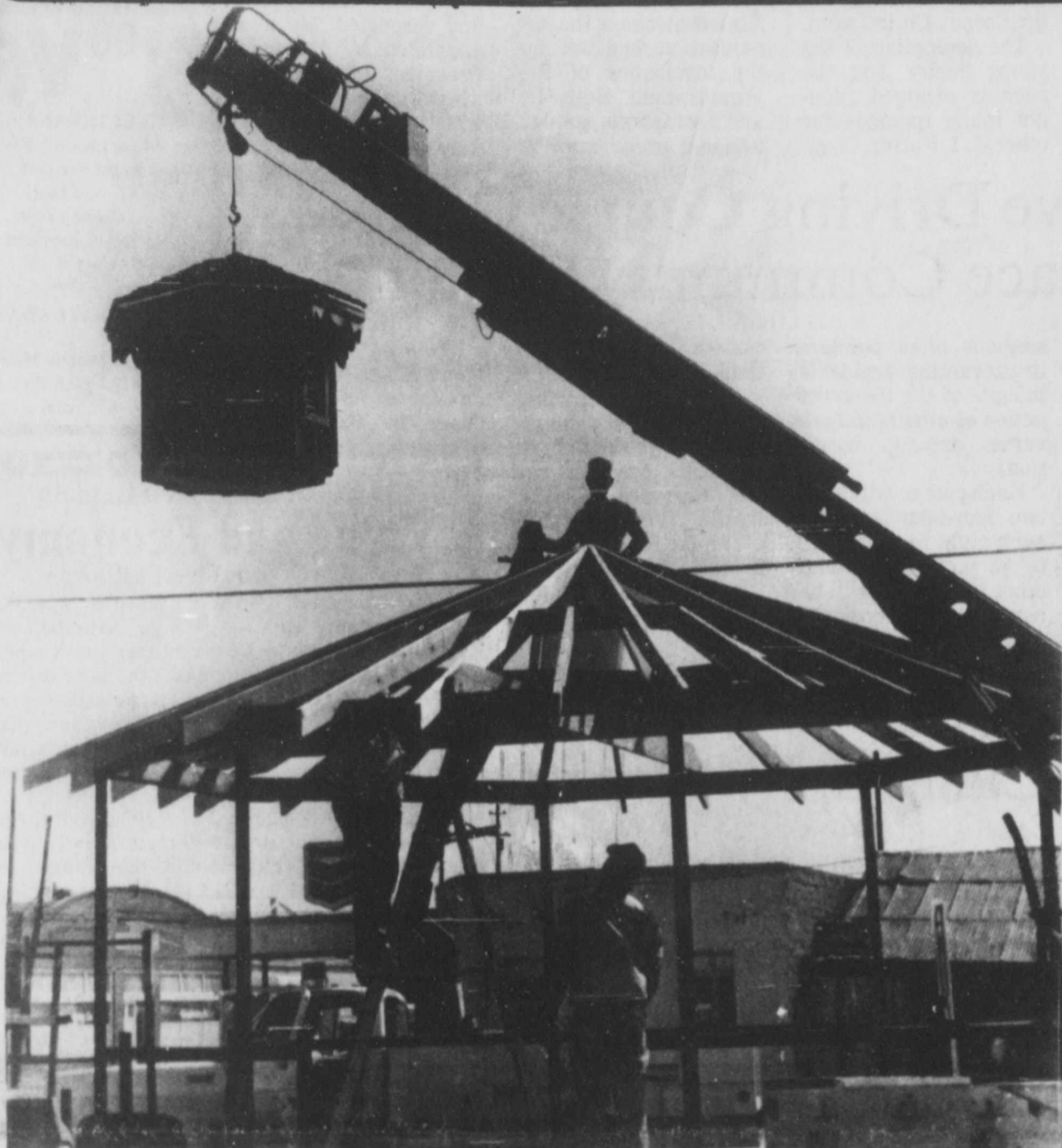
WORK ON THE BARBER PARK on 2nd Street continues. Tandy Curlee and Landmark Cablevision workers could be seen Friday morning placing the top on the Gazebo.
